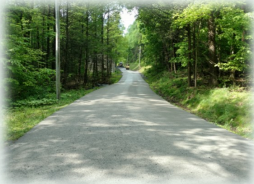
Driving Surface Aggregate (DSA) placed on Robinson Road Phase 3 in Jackson Township.
