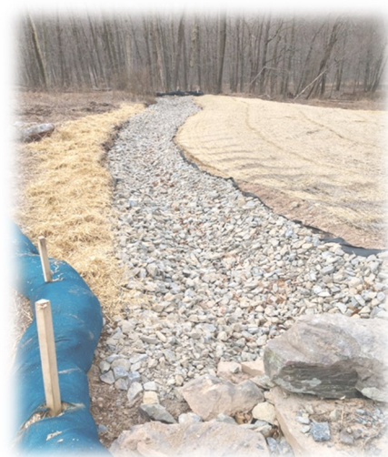
A newly installed rock lined channel on the PPL Rebuild Project in Carroll Township.
